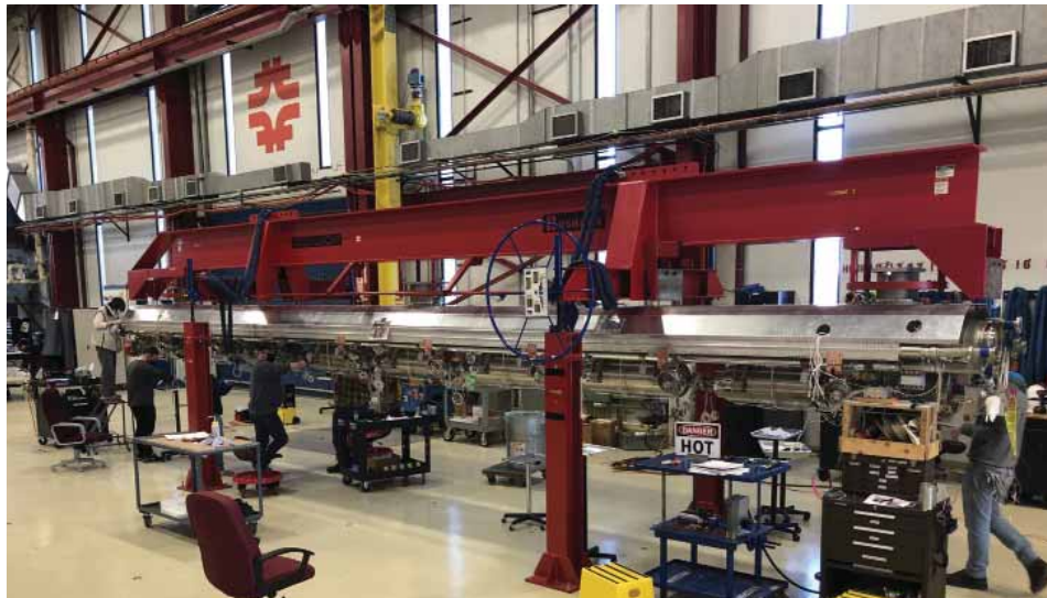
Assembly of verification cryomodule cold mass prior to insertion into the cryomodule vacuum vessel. Image: APS-TD process engineering group
