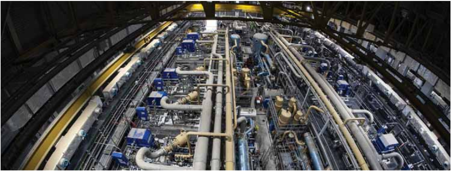
Over the past three and a half years, some 5,000 tonnes of equipment (tanks, compressors, piping, valves, truck-size electrical motors and Zeppelin-like gas bags) were installed in the cryoplant. Here, one of the three "trains" of helium screw compressors feeding the cold boxes with compressed helium at 20 bar. Image: ITER
